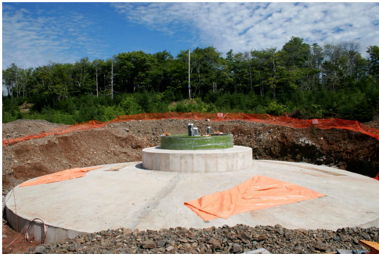
Figure 2-6: Finished concrete foundation for Natural Forces' Fairmont Wind Farm in Nova Scotia
